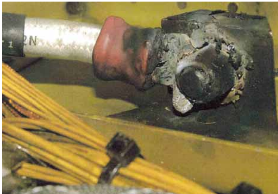
Figure 1: Corroded and burnt Earth Terminal
